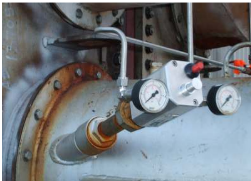
ACL 2000 installed on oil treater
